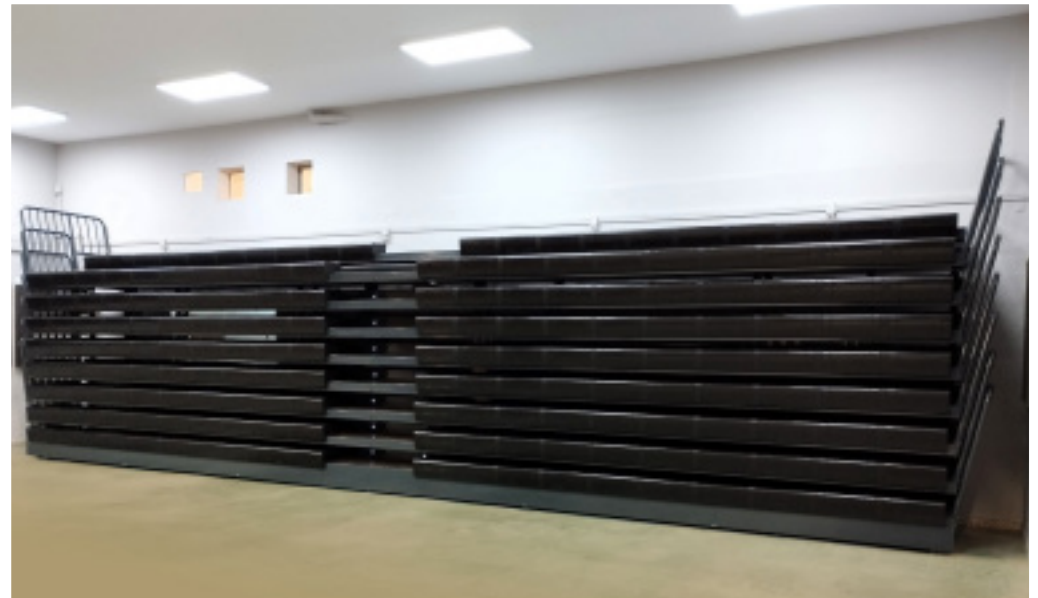
ELEVATED CONTINUOUS PVC SEATING
